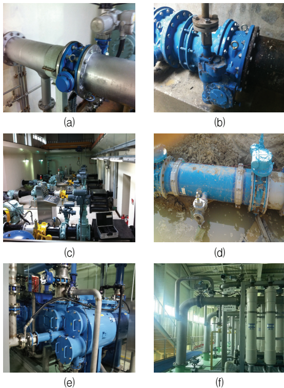
Fig. 6 Photos of the operating conditions for butterfly valves (a) drainage pump room (b) water pump room (c) filtration room (d) water pipe underground (e) reverse osmosis type of membrane device (f) micro filtration type of membrane device
