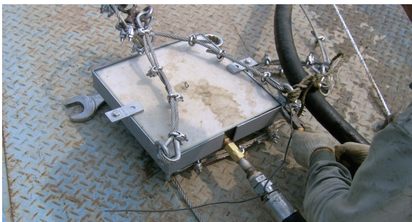
Fig. 2 Picture of water aeration
