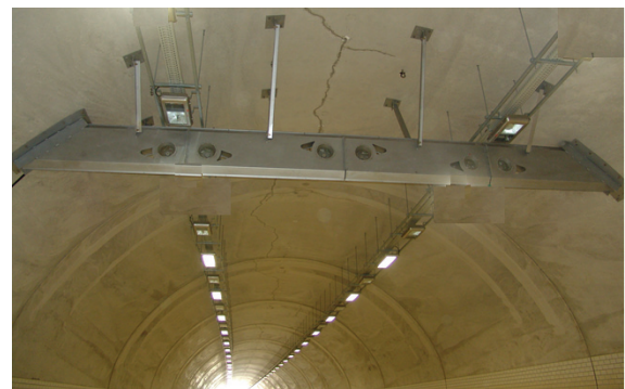
Fig. 5 Air curtain system in Maihyun No. 2 hiway tunnel
