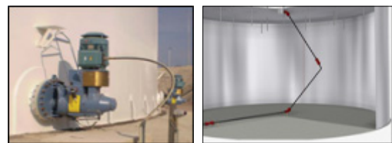
Fig. 1 Floating Roof Tank & Mixer
