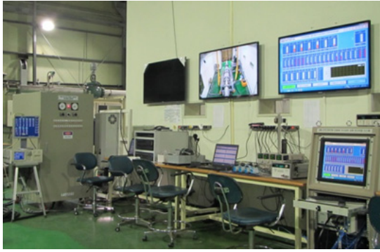
Fig. 8 Micro gas turbine control and monitoring room
