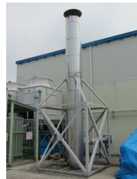
Fig. 7 Micro gas turbine exhaust duct
