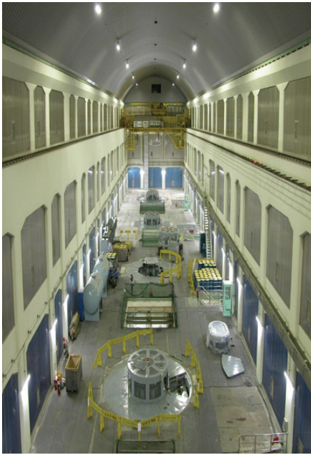
Fig. 5 Pumped storage power plant inside view
