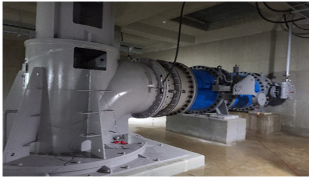
Fig. 7 View of rainwater pumping station
