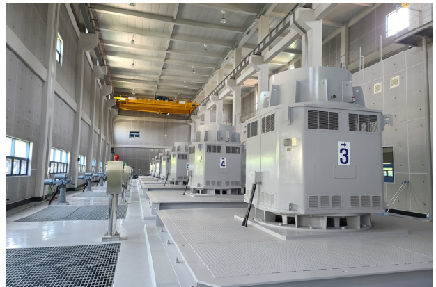
Fig. 3 View of rainwater pumping station
