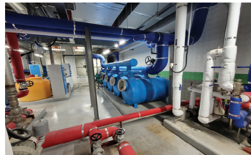
(b) Swimming pool machine room
