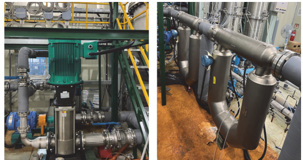
Fig. 6 Vertical multistage pump(Left), Coriolis mass flowmeter(Right)
