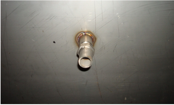
(a) Thermocouple on the ceiling
