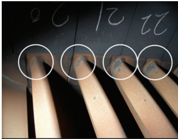
Fig. 1 Damage of 2 nd vane of gas turbine
