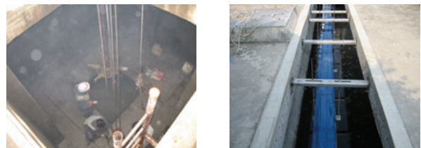
(a) Expansion of the inlet of (b) Increase of weir area the mixed basin
